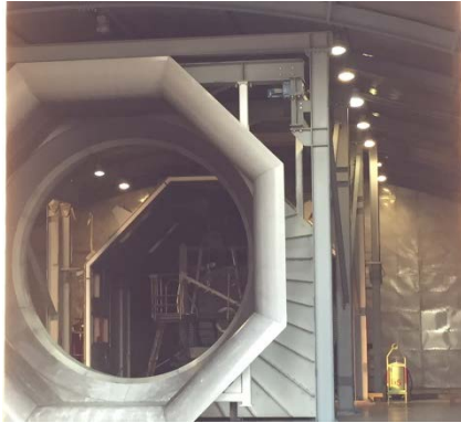
Enclosed Engine Noise Suppressors Hurlburt Field AFB, Florida
