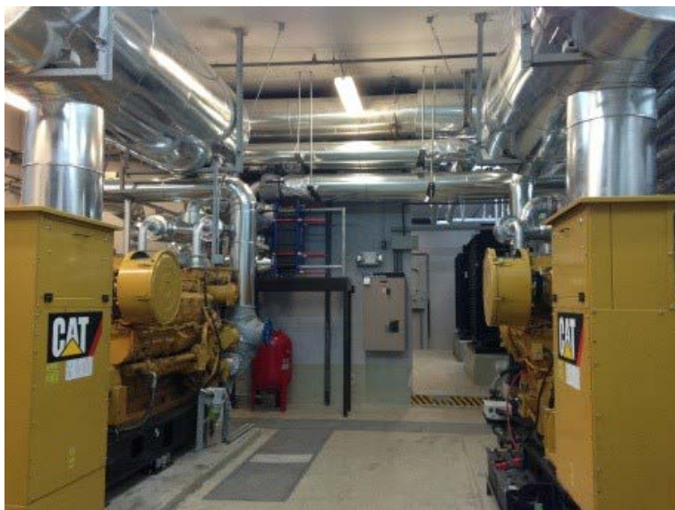
New Generator Plant Incirlik Medical Hospital, Incirlik AB, Turkey
