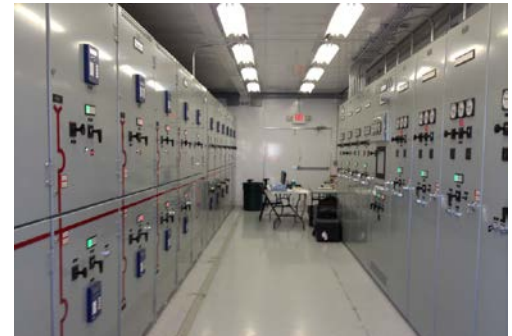
New Primary Electrical Substation David Grant Medical Center, Travis AFB, CA
