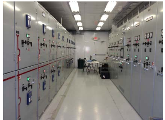
Hospital Substation, Emergency Power Supply David Grant Medical Center, Travis AFB, CA
